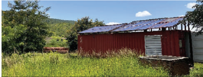
Solar panels powering the Kayelekera Health Centre
